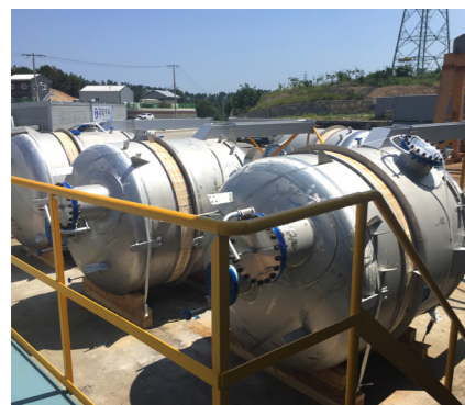
Reactor & Pressure Vessel
